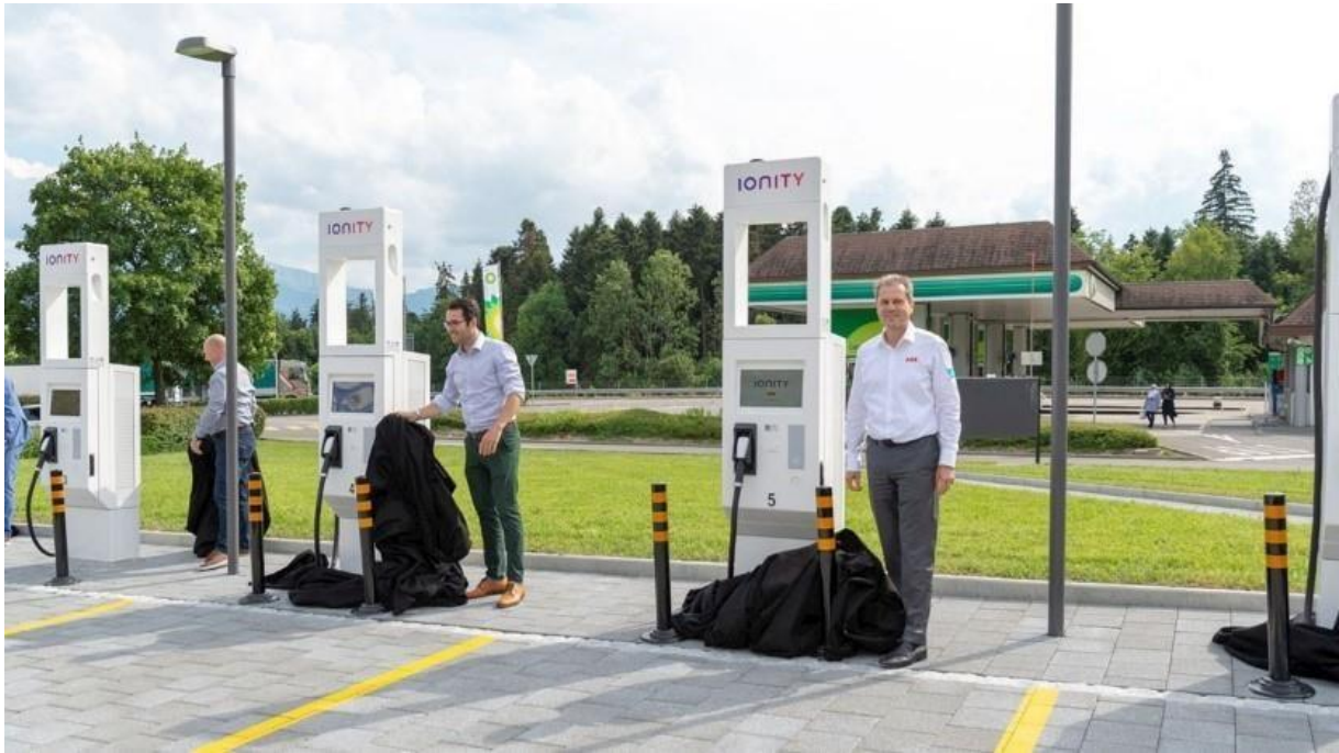
Ladestation IONITY. (Quelle: https://new.abb.com/news/detail/5227/abb-chargers-power-ionitys-opening-of-europes-highway-of-the-future )
